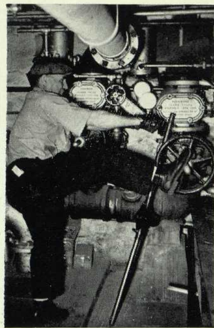
"Rollie" Snyder's really putting on the pressure here. Whenever you see someone up on a ladder or working on a steam pipe, you can make up your mind that Rollie is right on the job.
