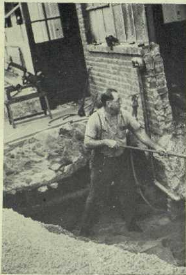
Erv lends a hand in preparing an underground bed for the oil storage tank recently installed in Plant II.
